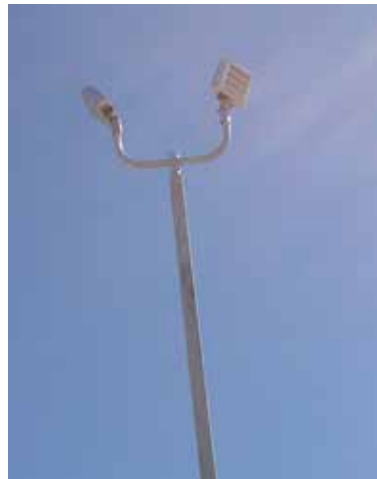
New LED Light Pole.
