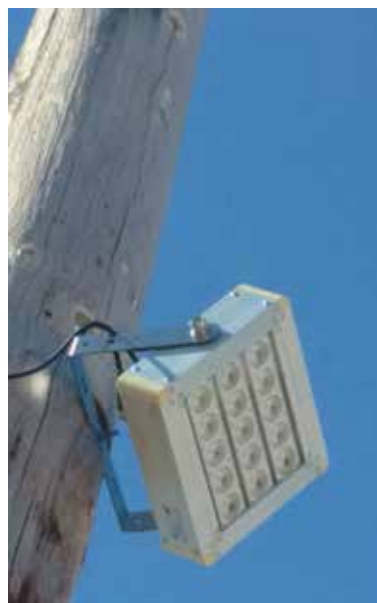
New LED Light Fixture.
