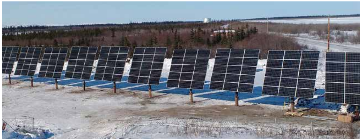
55 kW Solar PV Installation in Aklavik.
