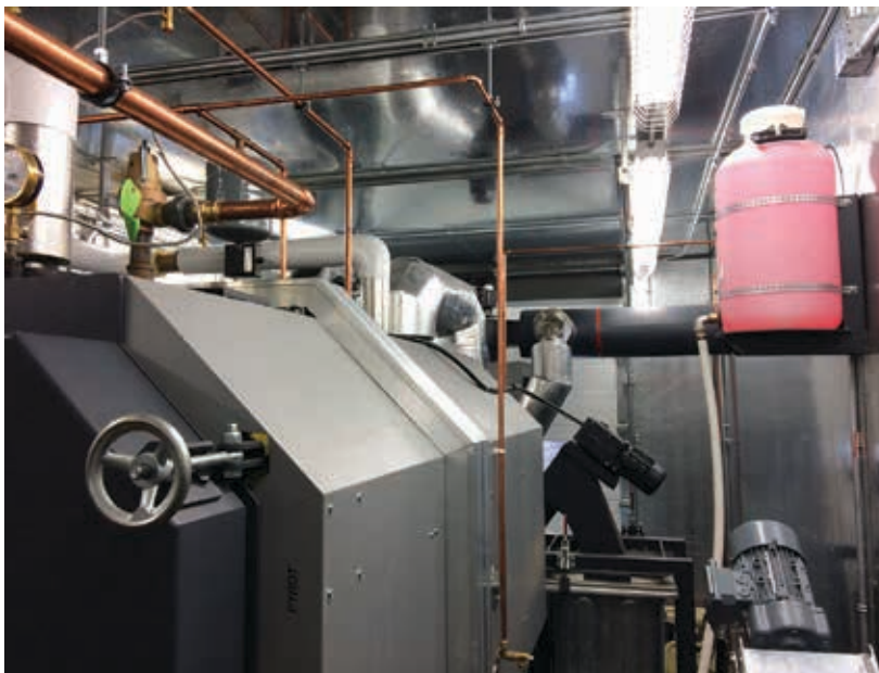
Prince of Wales Heritage Centre's biomass heating system upgrades make it more efficient.
