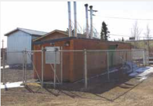
224 kilowatt wood pellet boiler at the Mackenzie Mountain School
