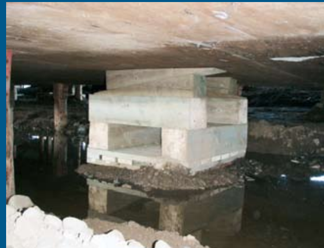
Wood crib blocking provides interim support for failed pile. Water must be drained to eliminate frost heaving.
