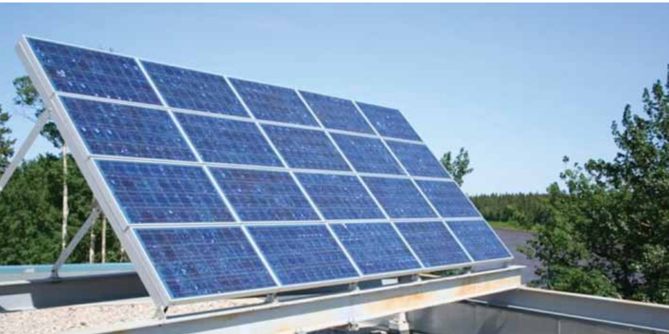
A solar panel located on the top of NTPC's Headquarters in Hay River.
