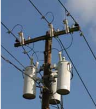
A power pole and transmission lines.
