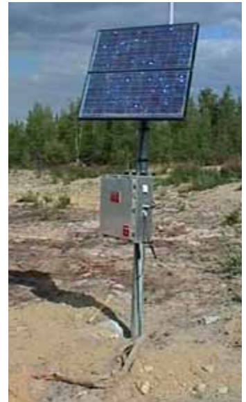
Solar panels at a Northern airport.
