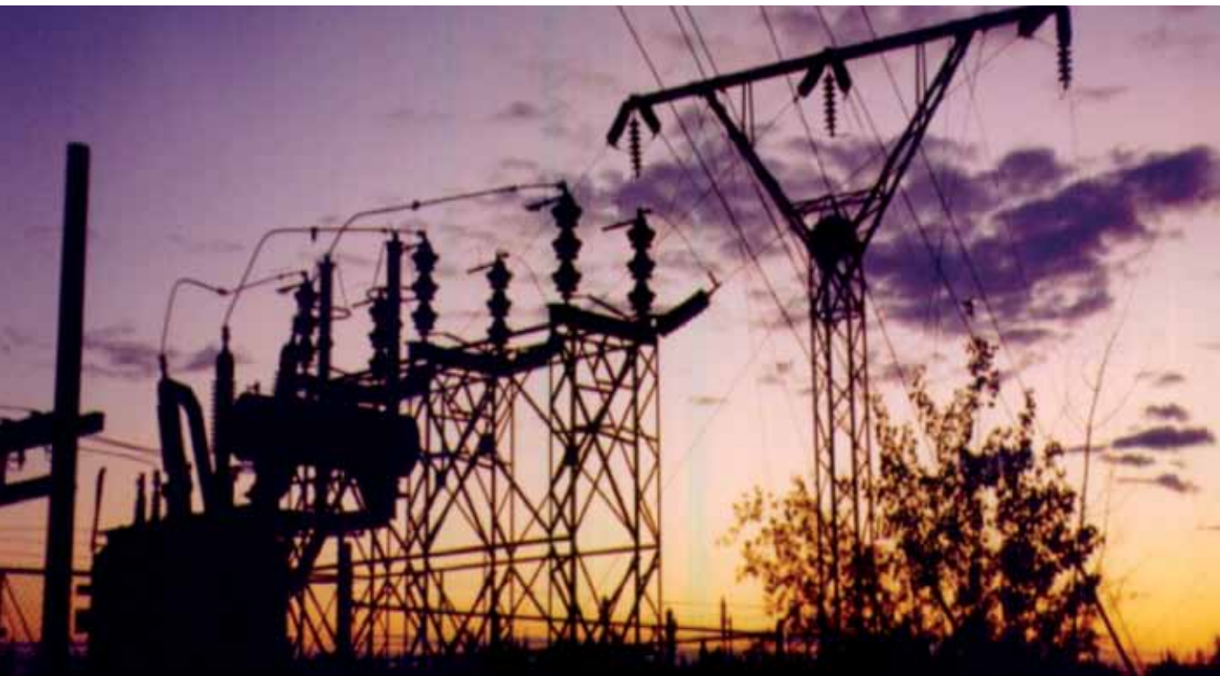
Transmission lines near Frank Channel.
