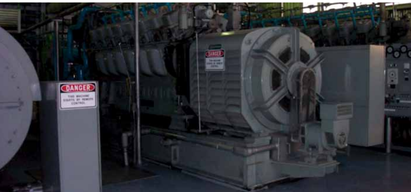
Generators at the Fort Smith power plant.
