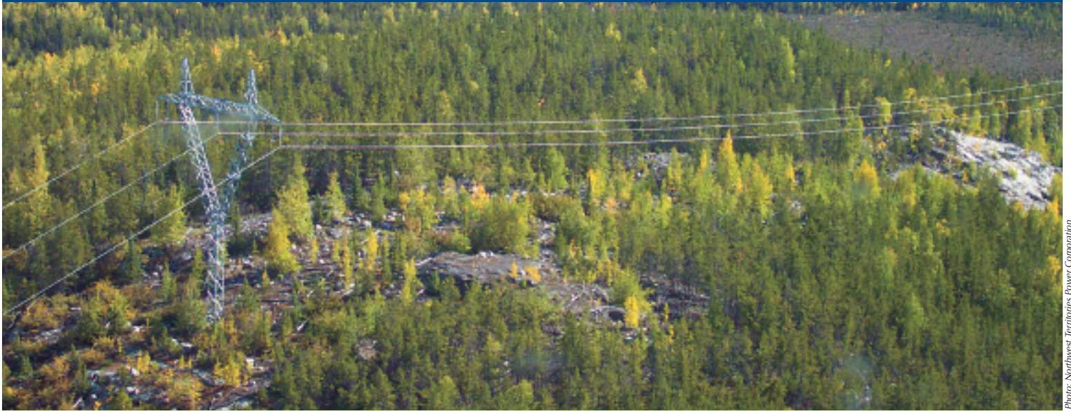
Transmission lines near Yellowknife
