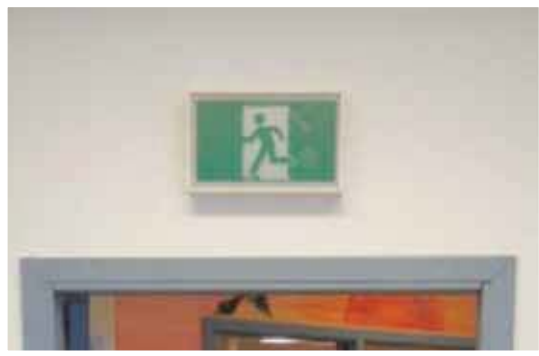
Exit sign at Moose Kerr School has been upgraded to code compliant LED exit light.
