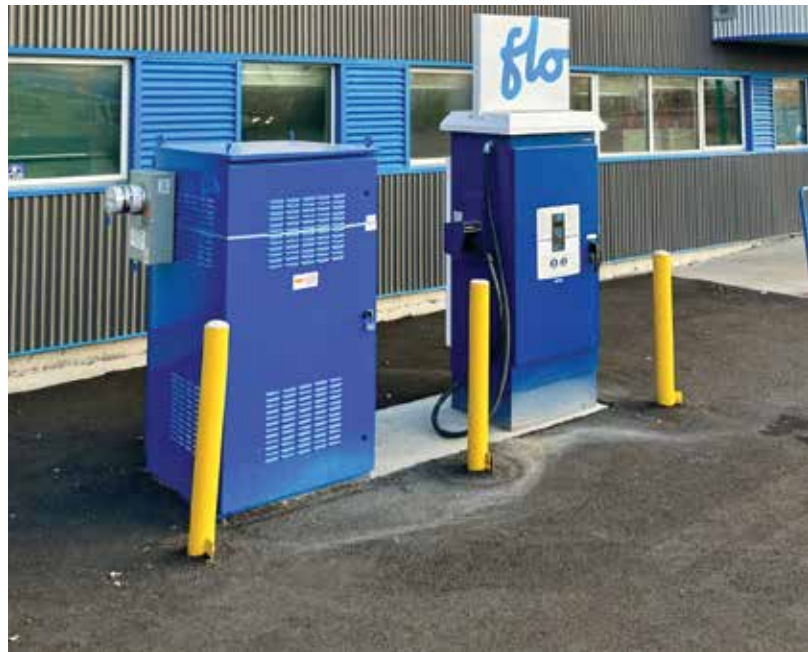
EV Fast Chargers Installed by Naka Power in Yellowknife
