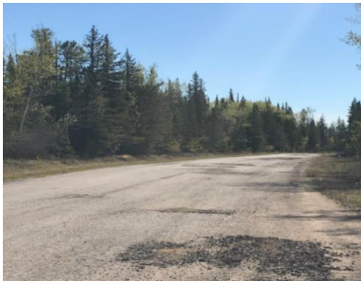
Curved section identified for resurfacing on the Hay River Golf Club and Ski Club Access Road.
