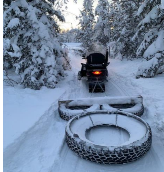
Trail construction and widening work underway on the community snowmobile and walking/skiing trail in Whatì.
