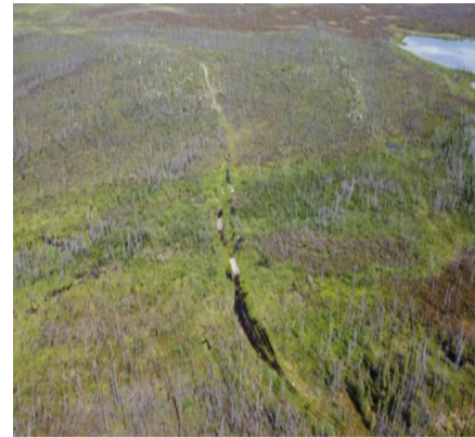
Aerial view of bridges constructed on the 3.6km community access ATV, snowmobile and Walking Trail to Secondary Beach in Whatì.
