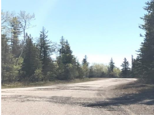
Section identified for resurfacing on the Hay River Golf Club and Ski Club Access Road.
