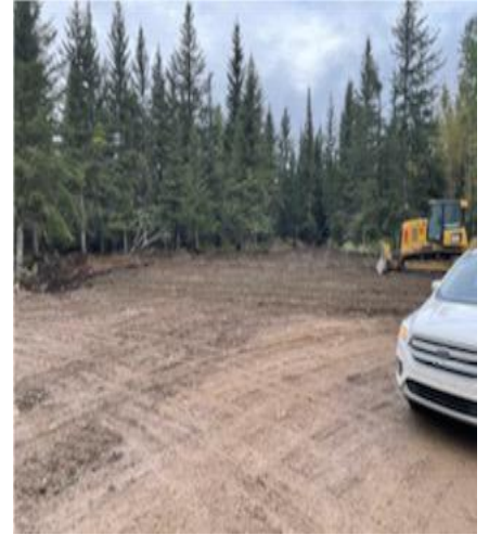
Construction work on the Nagel Channel Access Road and Boat Launch in Fort Resolution.
