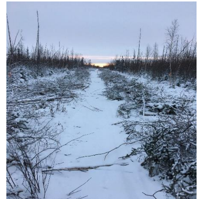
Construction underway along the new Four Mile Creek Quad and Walking Trail in Tulita.
