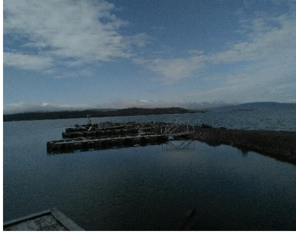
Łutselk'e Marine Facility after successful refurbishment of the three docks and the breakwater in Łutselk'e.
