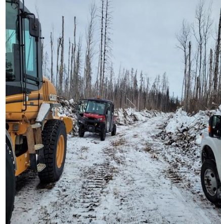
Construction underway on a section of the Cultural Camp/Community Camp trail in Kakisa.
