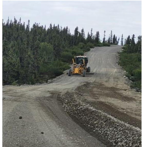
Grading operations as part of Summer 2021 continuation construction on the Wekweètì Access Road.
