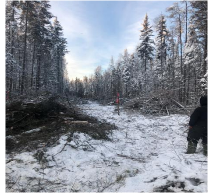
Phase I construction - Nahanni Butte Boat Launch and Boat Launch Access Road.
