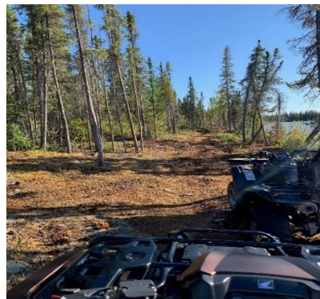
Construction underway on the 2.5 km community access ATV, snowmobile and walking trail to Lac La Marte in Whatì.
