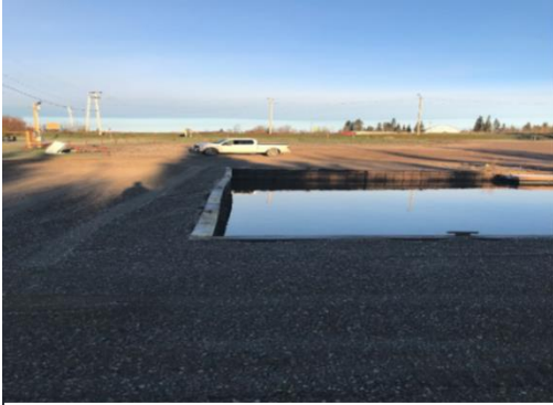
Porritt Landing Marina south shore retaining wall after completion of Summer 2021 continuation construction.
