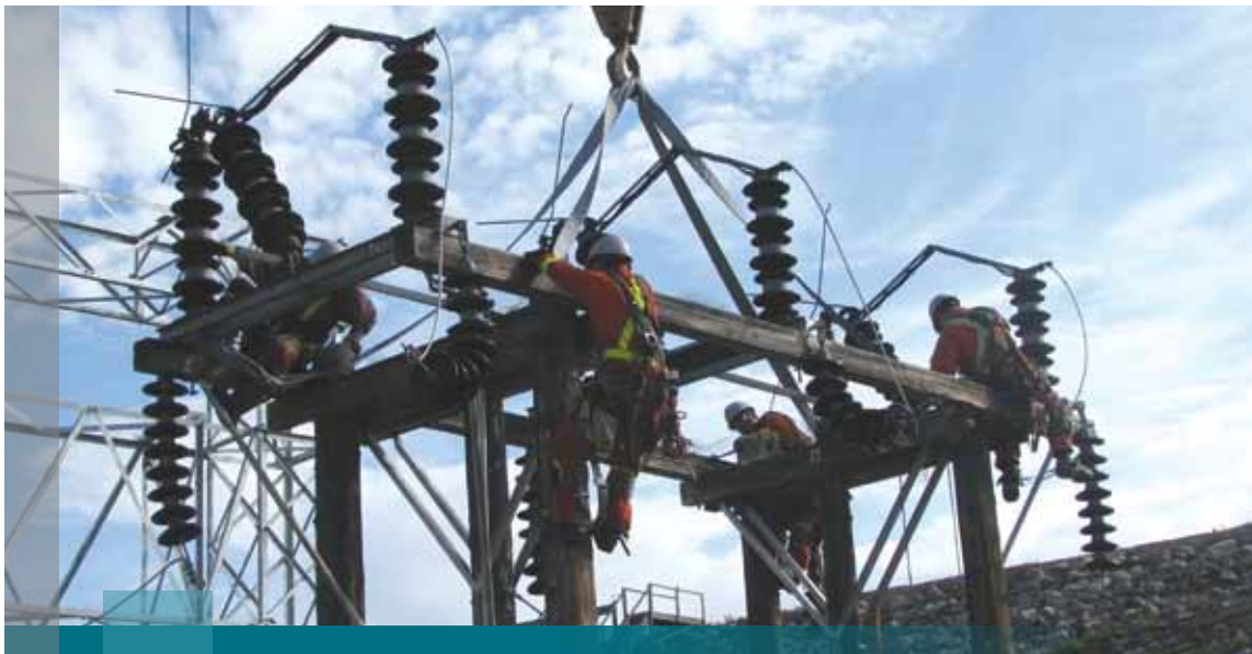
Construction of sub-station infrastructure by the Northwest Territories Power Corporation (Source: NTPC)
